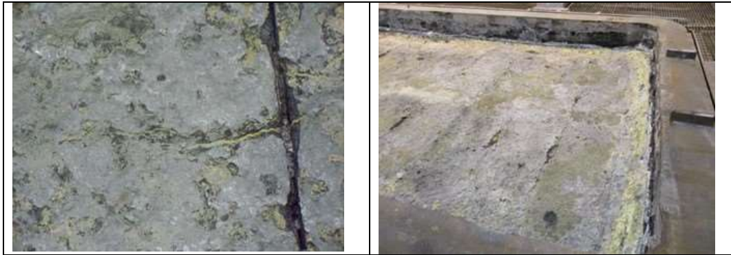
Figure 4. Cooling cracks on the top surface of the cathode panel.
